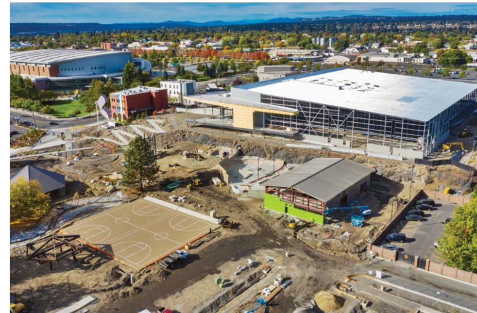
An aerial view of The Podium during construction looking towards North Spokane.
